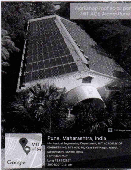
Solar panels on building roof
