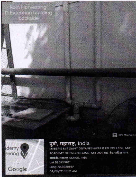
Rainwater Harvesting Tank
