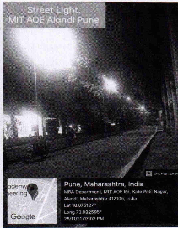
LED Street Lights
